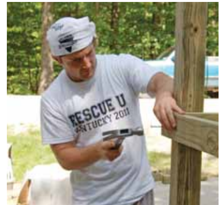
Rescue U volunteer Matt Murrin helps put it all together during a project in Morehead, Ky. Since its founding in 2006, Rescue U has completed about two dozen construction and repair jobs.
